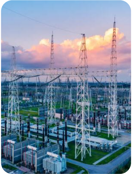
Substation & Smart Grid
