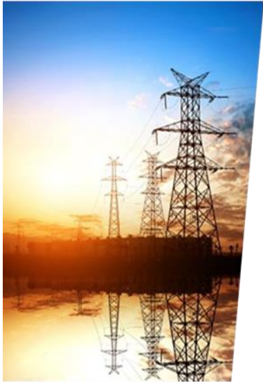
Substation & Smart Grid
